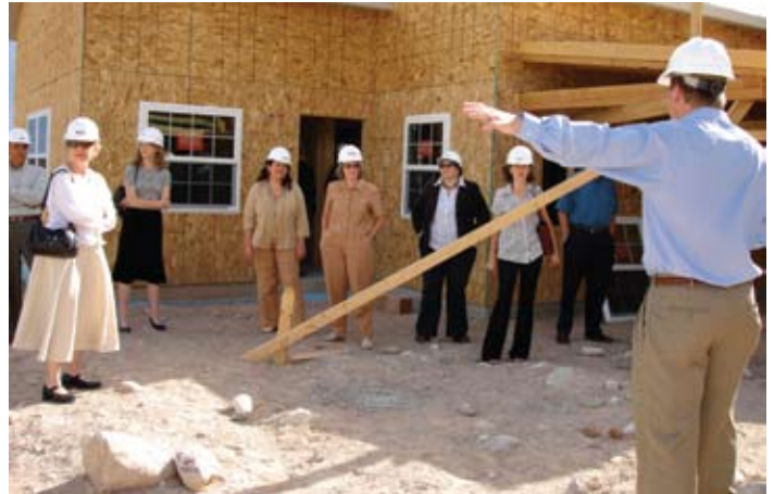
⋈ Tony Fox (right) gives board members and staff a tour of the new building construction.
